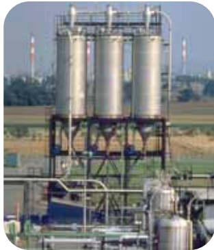
Storage at the Mont plant (Pyrénées-Atlantiques, France)
